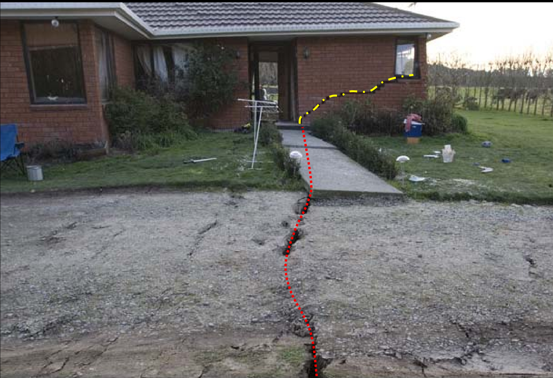
The Roberts house which was partially destroyed by the earthquake. Photo / Mark Mitchell
