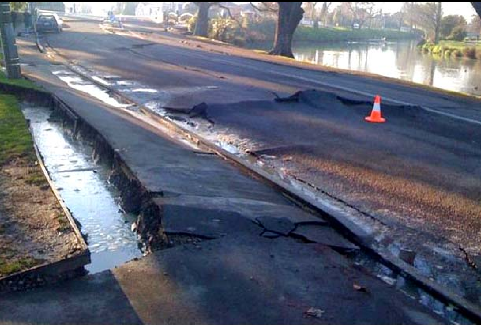
Road damage. Photo / Jemma Walker
