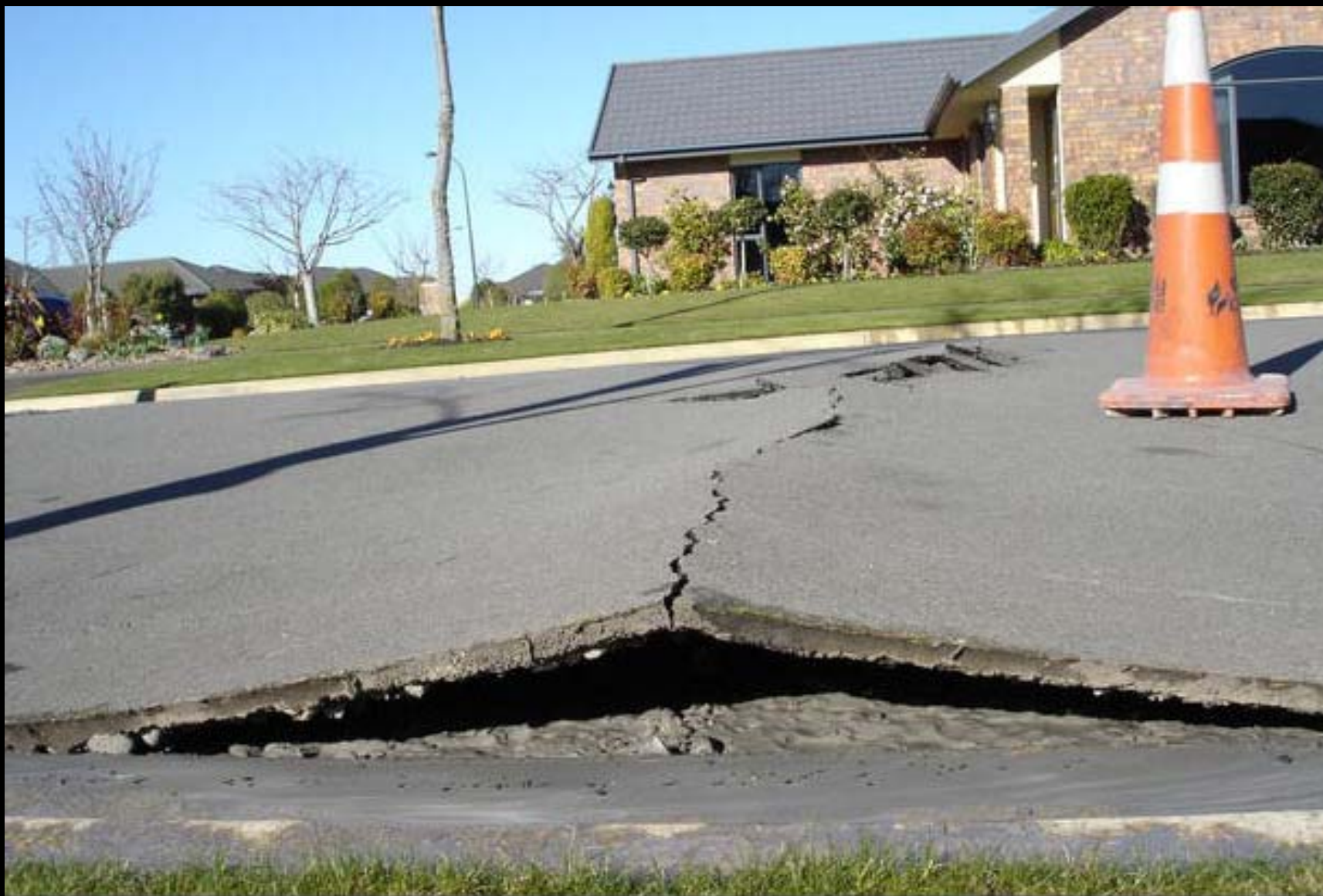
Road damage in Northwood. Photo / Keith Hitchings
